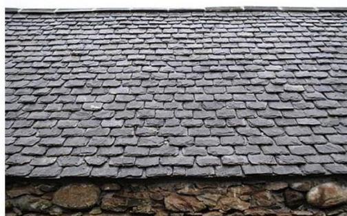
Close-up of restored Valentia Slate roof on historic outbuilding on farm near Waterville, Co. Kerry – a project funded under the GLAS TFB Scheme.
