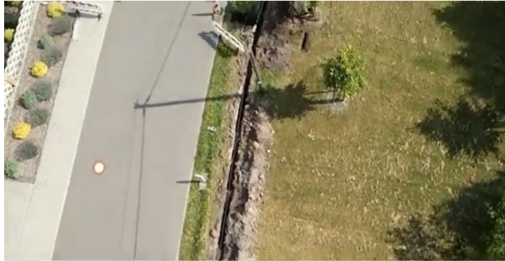
GRÜNEWALDE BECAME THE FIRST VILLAGE IN RURAL BRANDENBURG WITH A COMPLETE FTTH INFRASTRUCTURE
